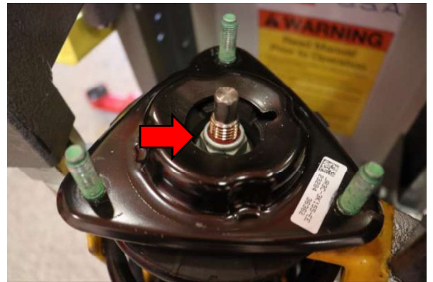
Step 16. Use a 21mm to remove the top hat mounting nut. Do not use an impact tool for this step, excessive rotation of the shock shaft during removal can damage the shock internal components. Hold shock shaft in place during nut removal to prevent damage.
